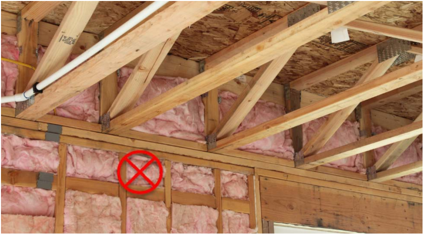
This photo shows rim joists that have been insulated. Unfortunately, the work is too sloppy to meet QII. There is too much compression and there are too many voids.
